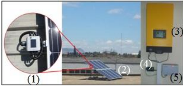
Figure 1: Photo of the photovoltaic plant localized at RMRE laboratory (Faculty of sciences, Meknès).
